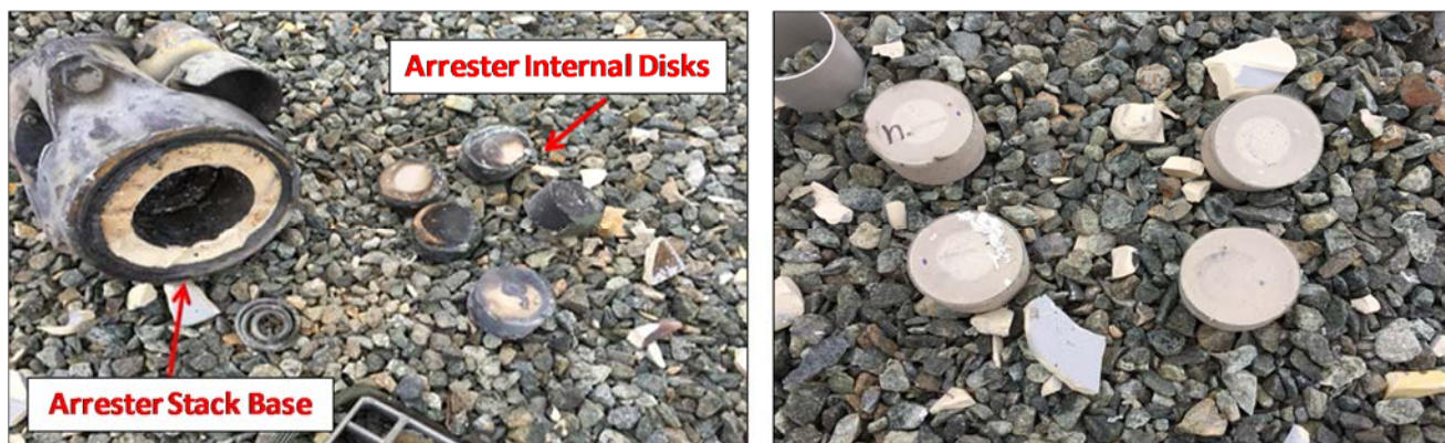
Figure 4: Internal MOV Disks from C-phase (left) and A-phase (right) Arresters
